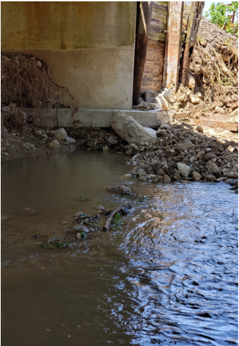
Twp Rd 178 Bridge Wash out below abutment
