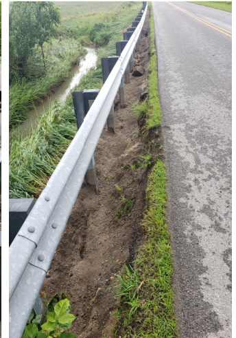
Washed out guardrail
